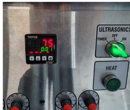
Figure 13 Generator Timer Running
