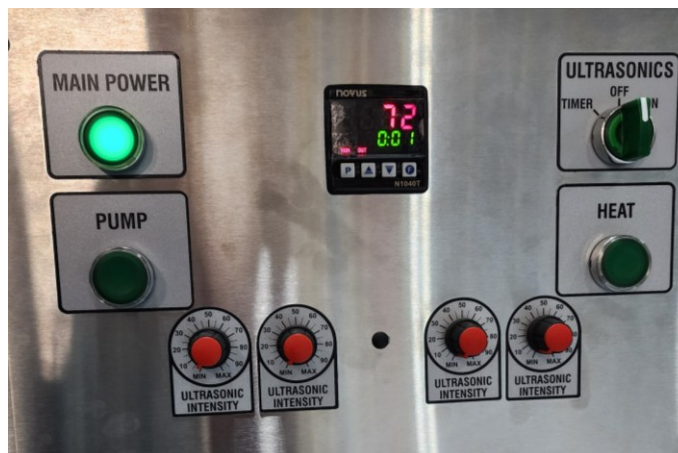
Figure 9 Ultrasonic Generators Turned Off
