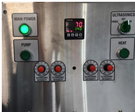
Figure 20 Pump Manual Control Off
