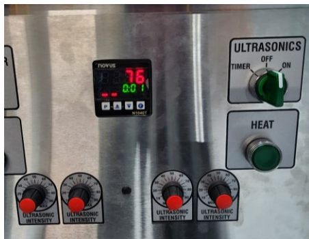
Figure 12 Generator Timer Off
