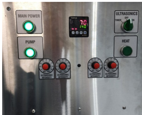
Figure 21 Pump Manual Control On
